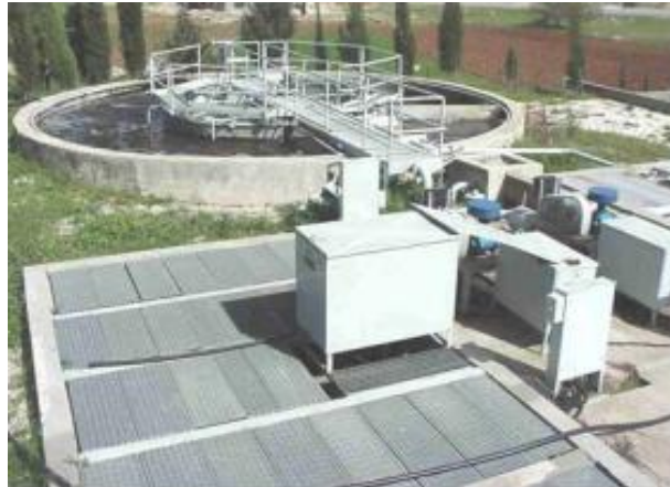
Photo 4: Birzeit water recovery facility through contact stabilization system
