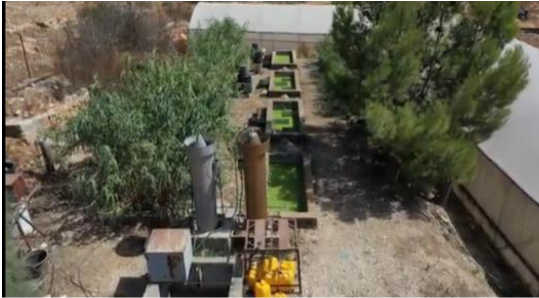
Overview of the pilot UASB-constructed wetlands system
